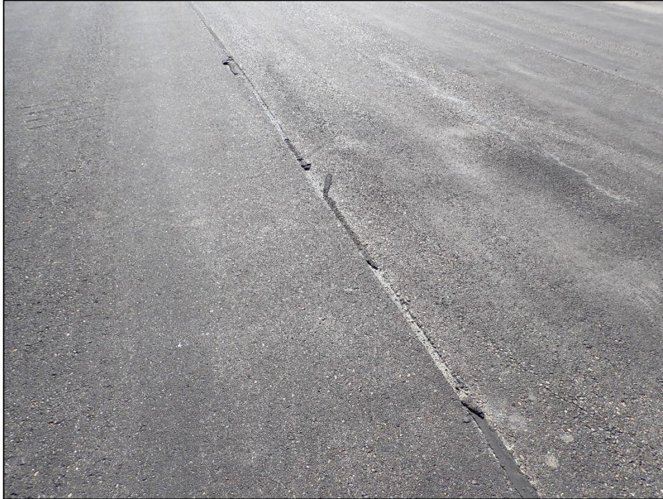
AP-11-09: L&T Cracking
