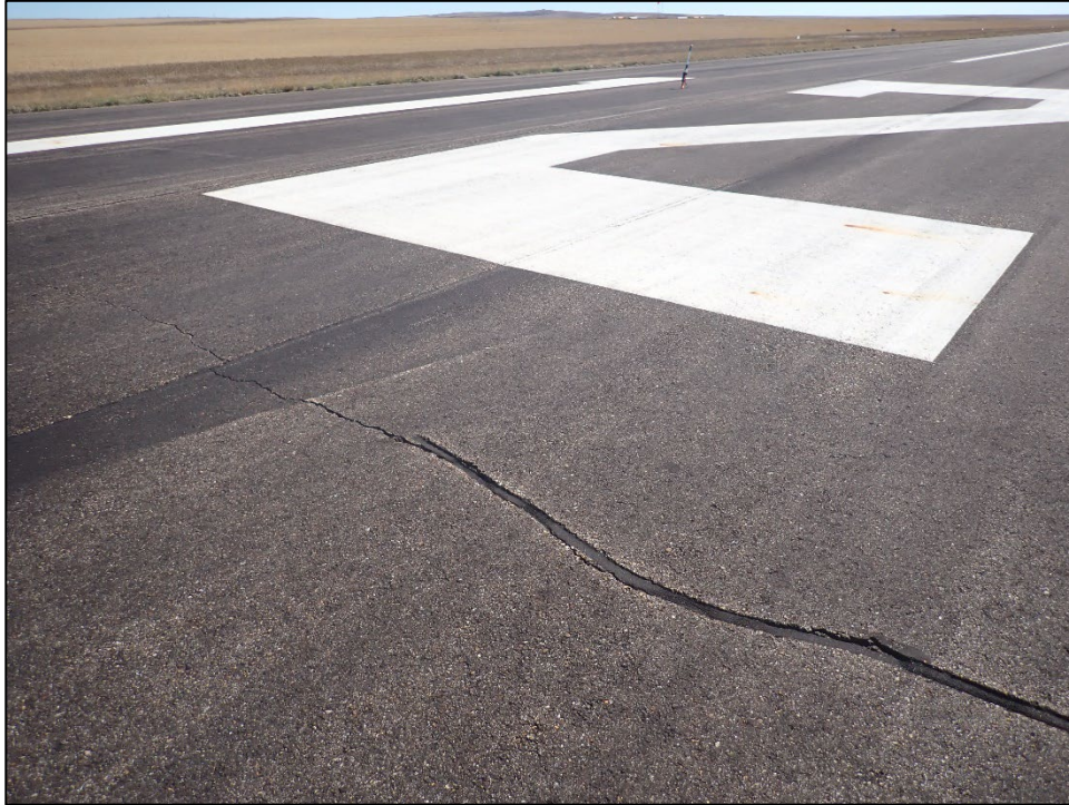
RW12-11-04: L&T Cracking
