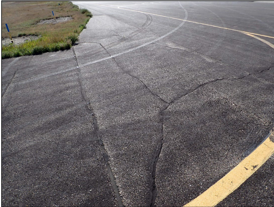
TW-11-02: L&T Cracking
