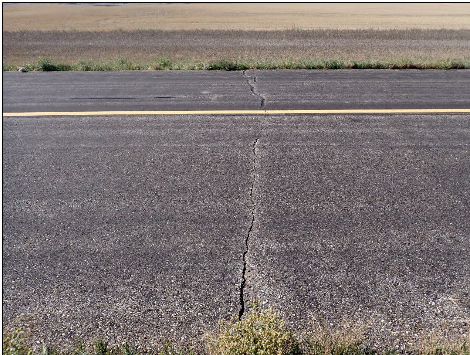
TW-11-24: L&T Cracking
